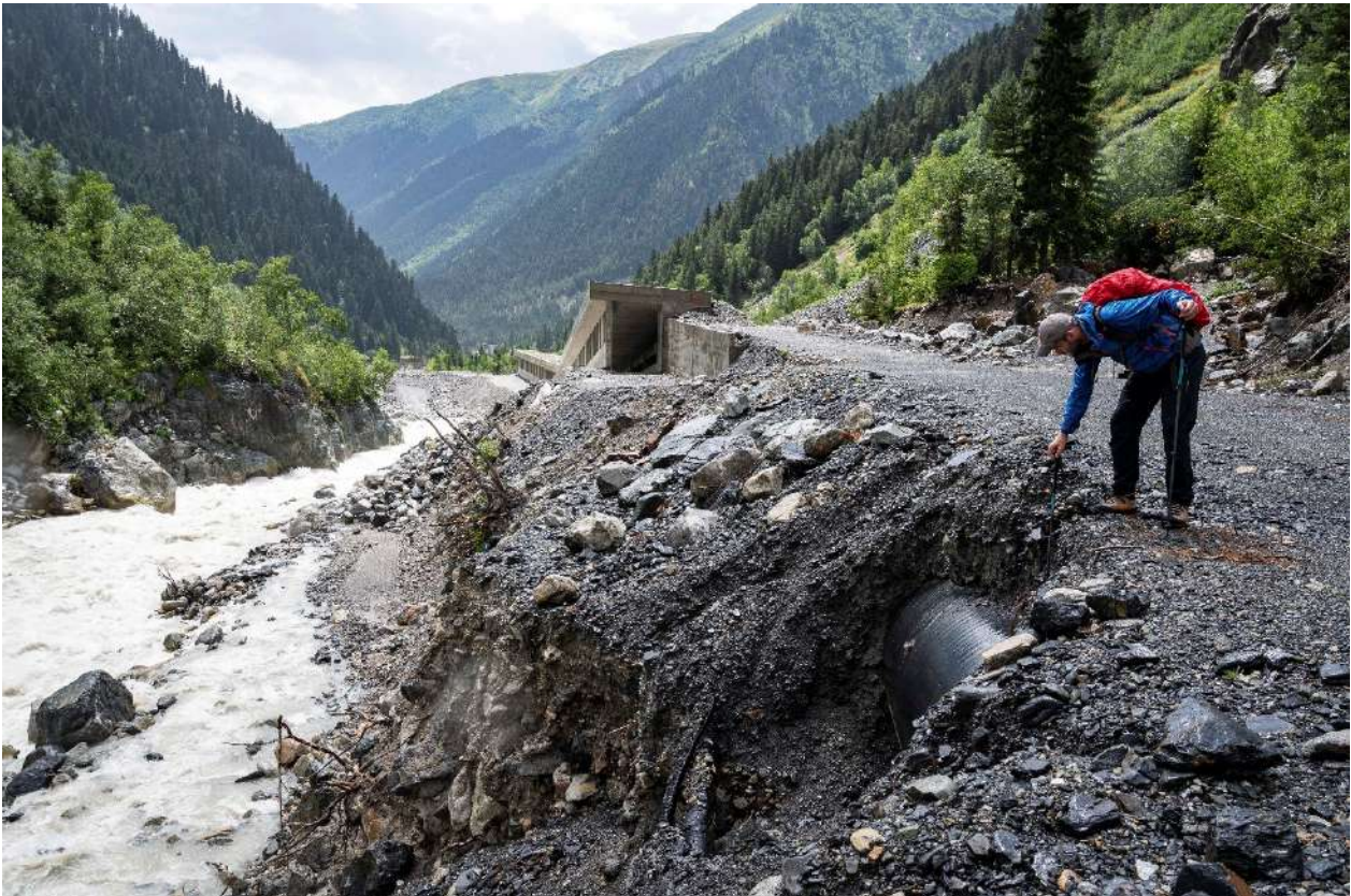
Fig. 7-4: The exposed penstock is located directly at a bend in the channel (317048/4776420). Due to the discharge in the riverbed, this location is particularly susceptible to possible erosion (Photo by Resinger 2020).
