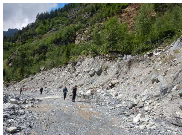
Fig. 4-11: Cut slope of construction road within the debris cone of deposition area M-D5a. View to the southwest.
