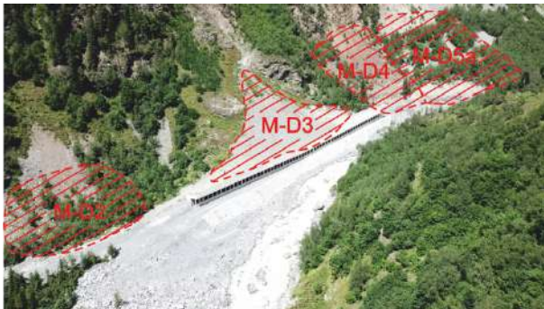
Fig. 4-2: Deposition areas M-D2, M-D3, M-D4 and M-D5a adjacent to the gallery, view to the north.
