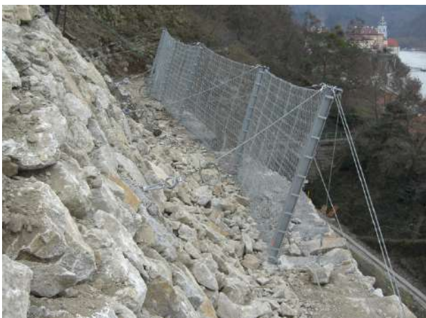
Fig. 12-1: Technical rockfall protection fence (2,000 kJ) on a dam embankment
