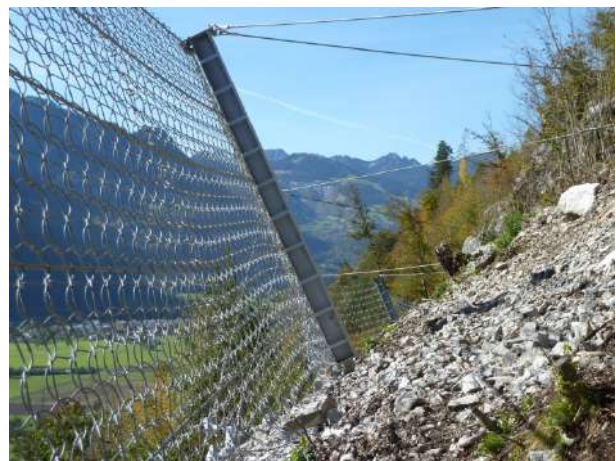
Fig. 12-2: Technical rockfall protection fence (2,000 kJ) on a natural slope
